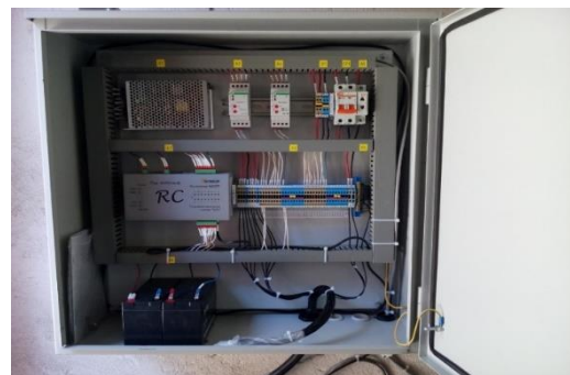
Fig. 6. Set of telemechanics from the transformer station
