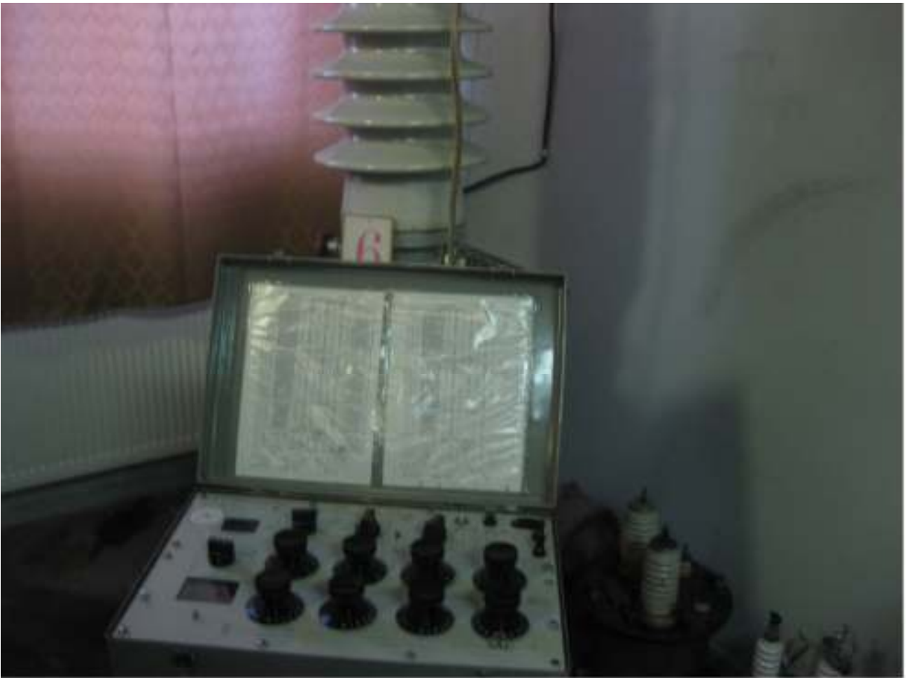
N.6 Determining high voltage bushings insulation systems dielectrical loss and capacity by standard method
