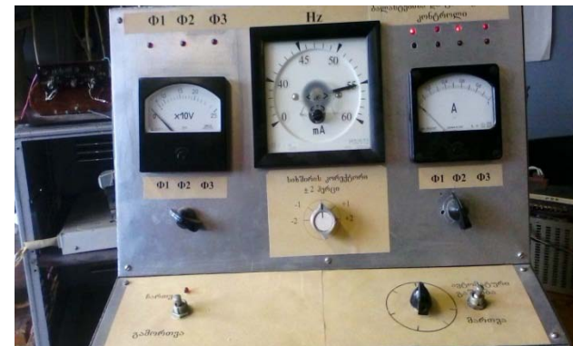
Regulator of hydroelectric aggregate frequency
