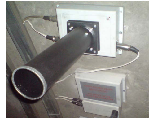
The ventilation control system of Chakvi-Makhinjauri tunnel.
