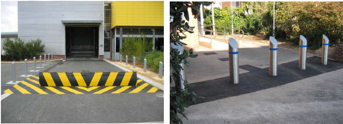
Figure 2 - Anti-RAM Barriers to prevent penetration of vehicles
